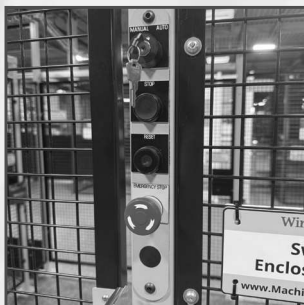
Switch Enclosure Post
